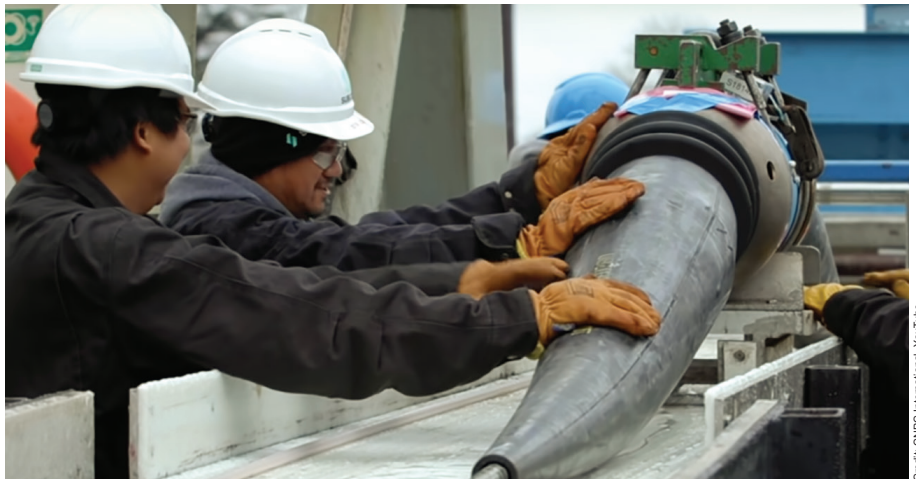
Workers position a submarine fiber-optic cable for installation. Concerns that the global submarine cable system may be used to conduct espionage is driving a clash between China and the United States.
