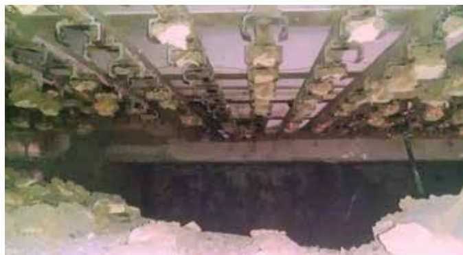
In extreme catastrophic ceramic anchor failure cases, refractory sections can fall out and leave major gaps or holes in the lining.
