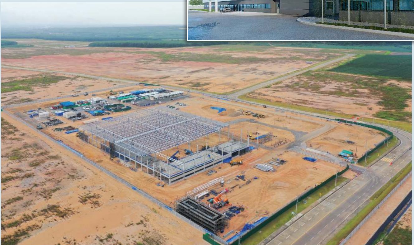
Top: A rendering of CoorsTek's finished plant in Thailand. Bottom: Construction proceeds on CoorsTek's Thailand plant. Credit: CoorsTek Inc.
