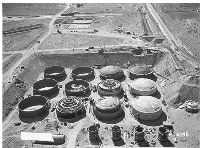
Figure 1. 1943 construction of nuclear waste tanks at the Hanford site. These tanks were designed with a 20-year lifetime, although some waste (including the waste stored in the above tanks) was later relocated to tanks with a 50-year lifetime. 1
